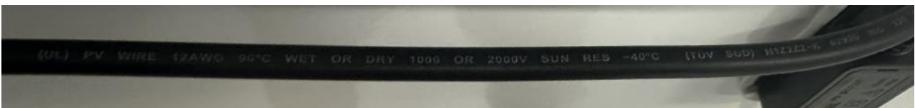
View of cable
